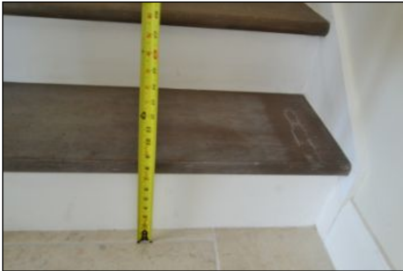
Rise is too tall at bottom of steps
