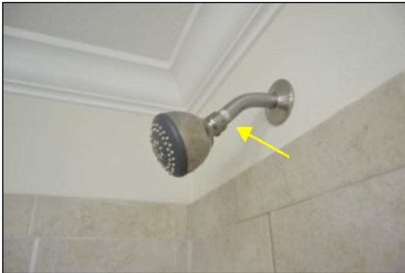
Leaks at shower head
