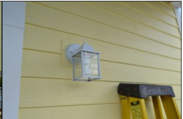
Light fixture has no power ( right of entree door)
