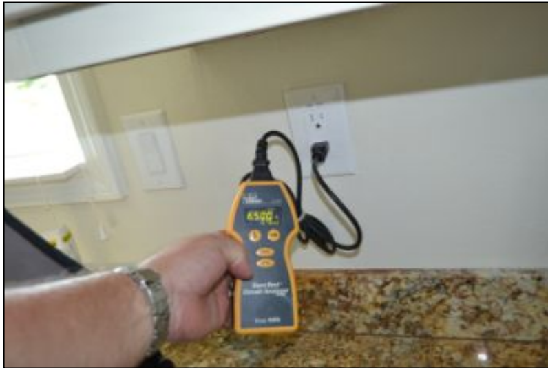
Kitchen GFCI failed trip test
