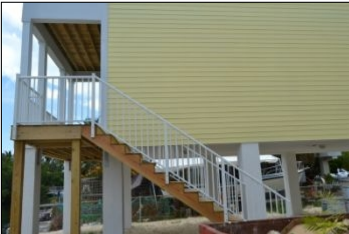
Missing light fixture above the stairs
