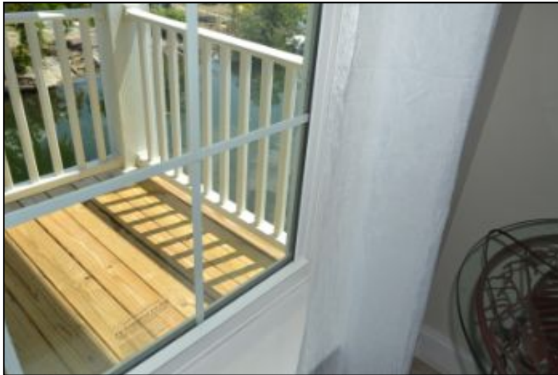
Missing window screens at several windows
