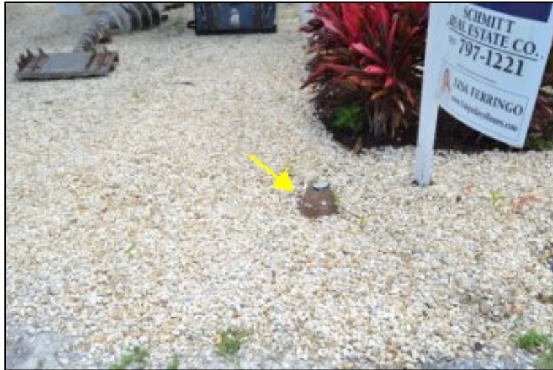
Meter is recessed below grade
