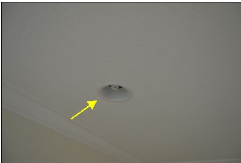
Three way switch and stair light not working properly.
