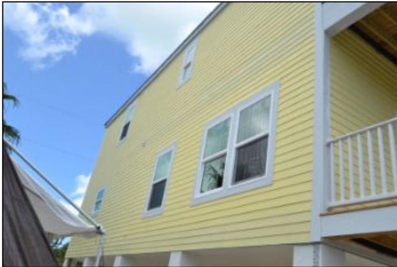
Missing gutters observed / overhang less than 6"
