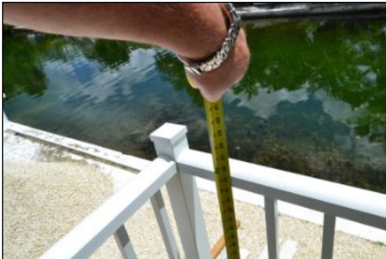
Exterior rails are 1/2" low.
