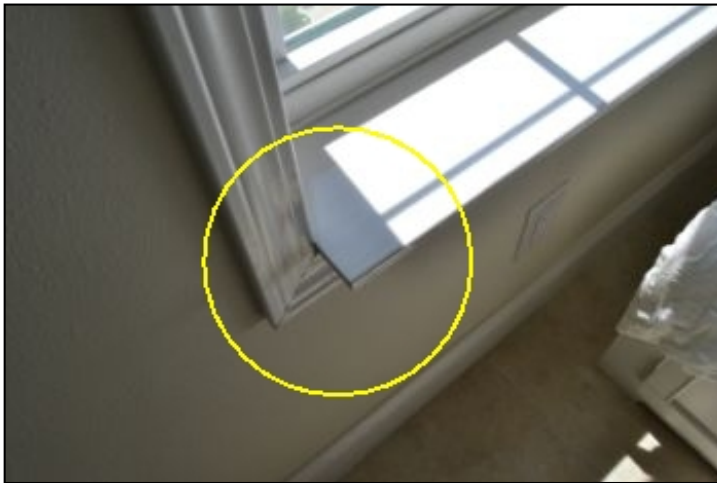
Sills are too big / unsupported overhang
