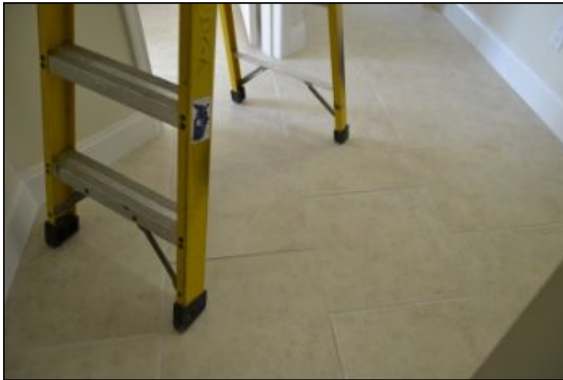
Uneven floor tiles
