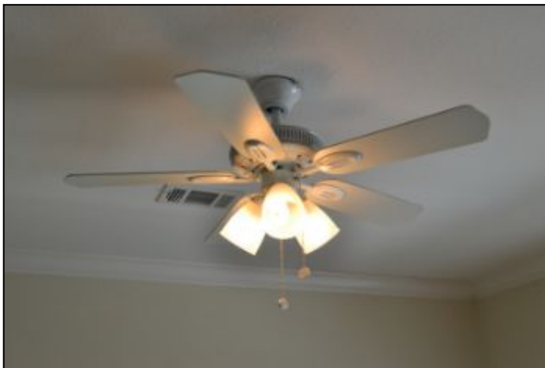
Living room ceiling fan is not working properly.
