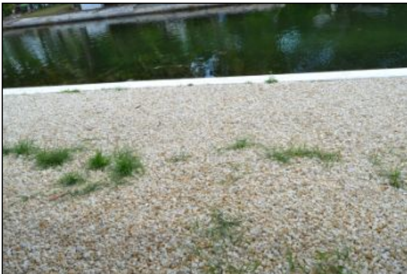
Improper grading toward the canal. Swale needed.
