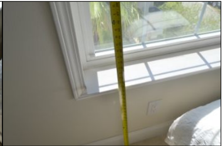
Sill heights are less than 36" / no fall protection at windows.
