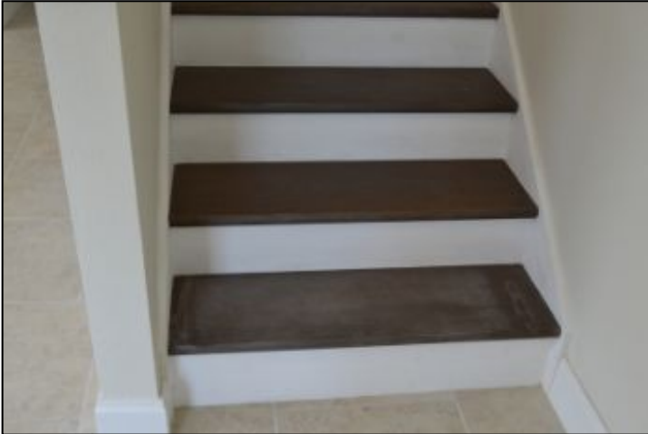
Damaged tread finish
