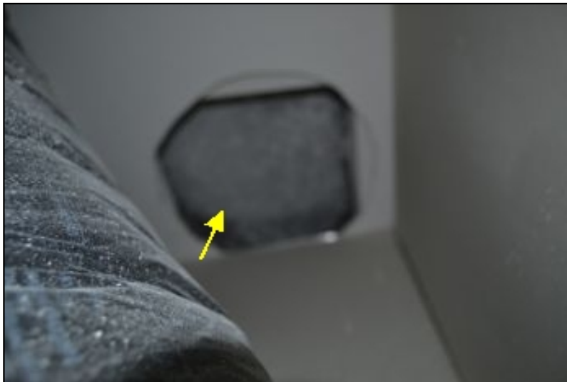
Hole in AC closet ceiling
