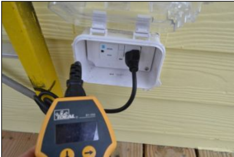
GFCI at right of entree door would not reset.
