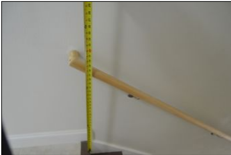
Stair railing is mounted too low, must be 34"-38"
