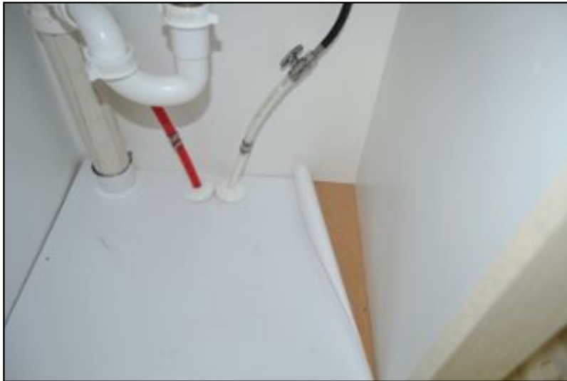
Delamination at bath cabinet
